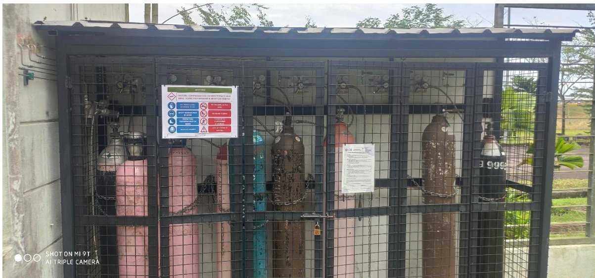
Picture 1: Safety signage for gas house
